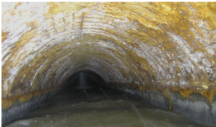
Exposed Reinforcement/Rebar (P-219-085-768-869)
