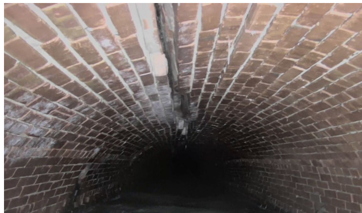
Missing Bricks and Mortar (P-217-081-373-915)
