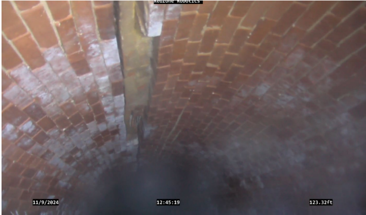
Cracked Brick Pipe Crown / Missing Bricks (P-217-081-373-915)
