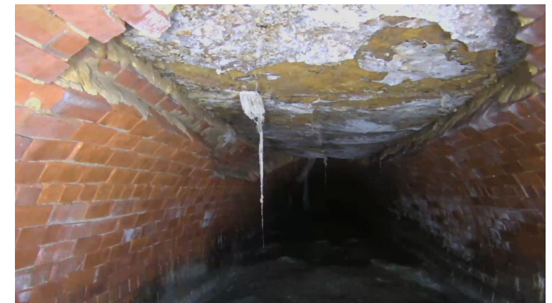
Previous Repair Corroding (P-217-079-070-494)
