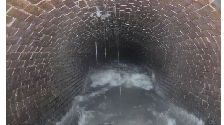
Water Intrusion/Infiltration (P-217-082-933-620)
