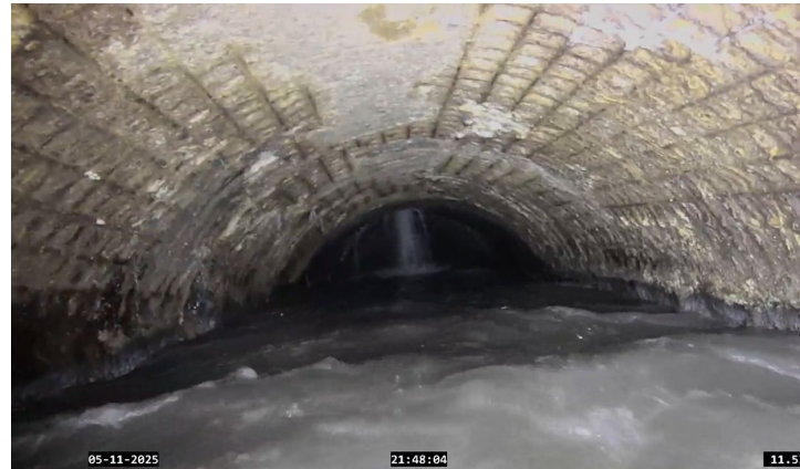
Exposed Reinforcement/Rebar (P-218-084-869-929)
