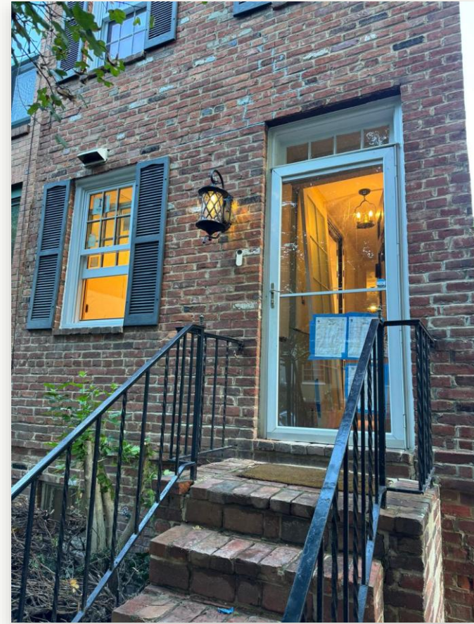
Close-up — current door condition
